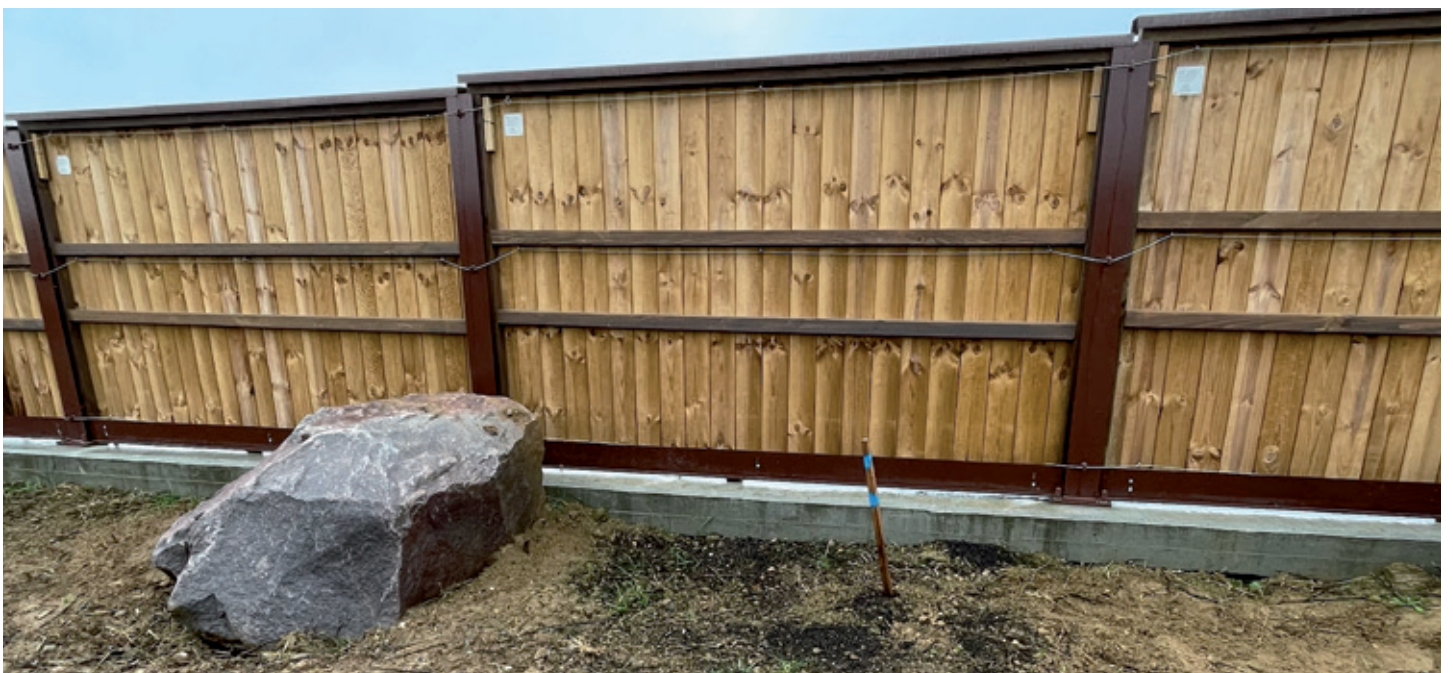
Figure 13: On the western bypass of Strasbourg, the panels are linked together by a metal cable and connected to the top of the metal posts. In the event of a possible breakage of one of the panels, this prevents them falling onto the roadway (4 mm diameter stainless steel cable). ©VINCI Autoroutes.
