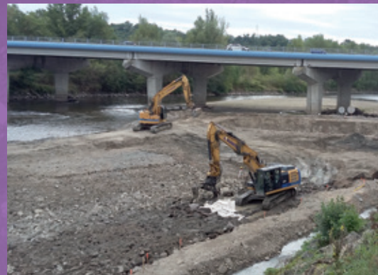
Figure 41: The works were carried out progressively from one bank to the other, in the riverbed upstream of the weir and requiring the displacement of large blocks for the formation of the ramp. ©VINCI Autoroutes Photo Library
