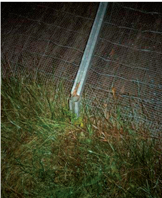
Figure 15: Broken posts of a fence fitted with heather panels after Storm Ana in 2017. ©VINCI Autoroutes.
