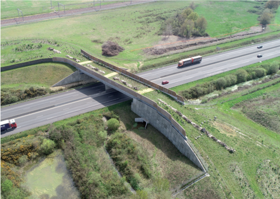
Figure 14: Case of an embankment structure (Bas-Bry - Cofiroute). The sight screens on the structure extend outside, beyond the wing walls and at the start of the access ramps for approximately 15 metres on both sides of the structure. ©VCT.
