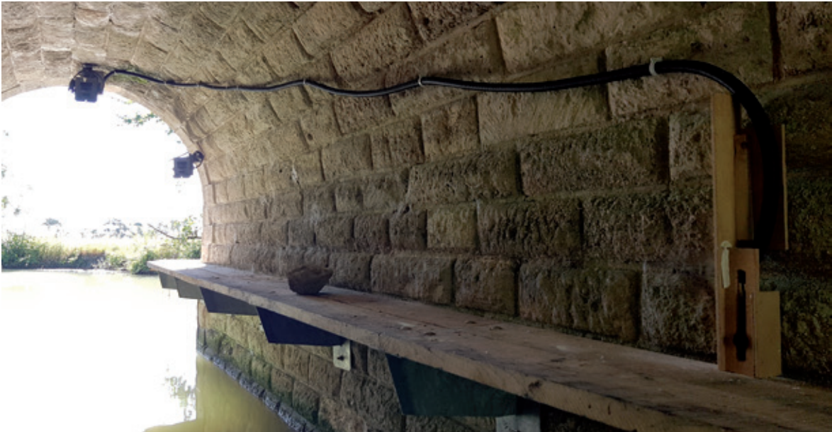
Figure 76: Infrared barrier detection system triggering a camera trap on the corbel of a motorway hydraulic structure. ©LIFE VISON/LPO France.
