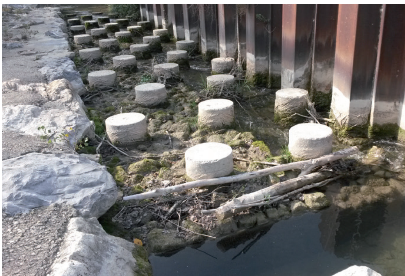
Figure 50: Jam at the entrance to a fish ramp, making the adapted structure unusable by fish ©VINCI Autoroutes Photo Library
