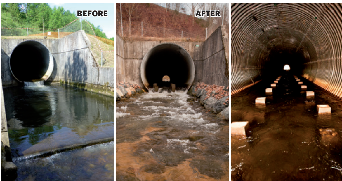
Figure 83: Presentation of the culvert before (left) and after works (centre and right). Source ASF.
