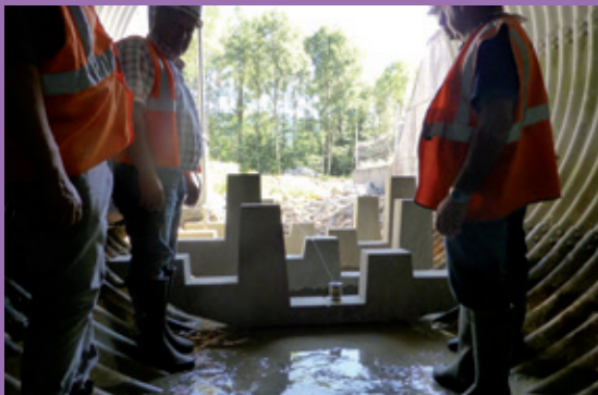
Figure 37: Setting up large rough elements in the bed of the structure to reduce the flow speed and create rest areas for fish. ©VINCI Autoroutes Photo Library
