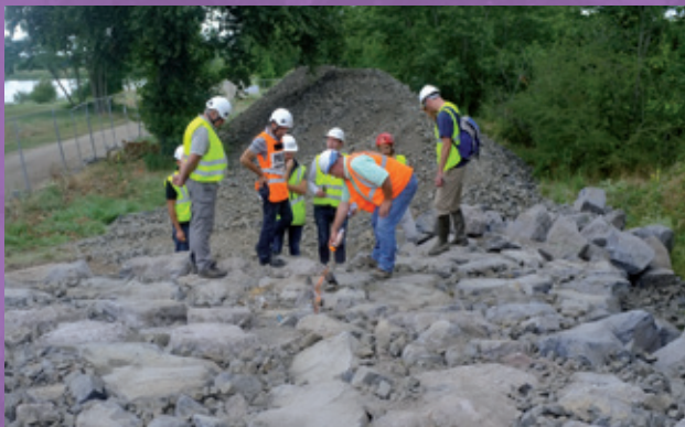
Figure 40: Making a test strip for the creation of a ramp for fish and canoes to pass. ©VINCI Autoroutes Photo Library
