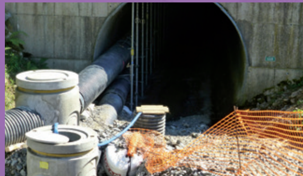
Figure 38: Setting up cofferdams and diverting the river to be able to work in the dry. ©VINCI Autoroutes Photo Library
