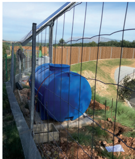
Figure 20: Setup of a holding tank fitted with a solar panel and supplied by a borehole. ©X-AEQUO.
